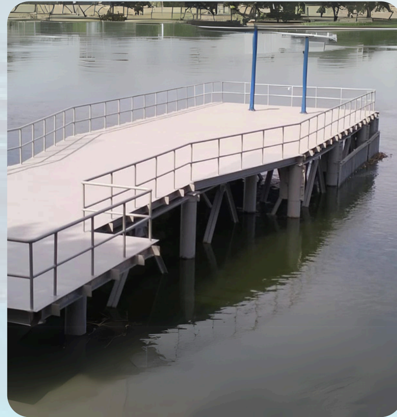
Installation of Assiut water station suction pipes -Installation of clamps and iron beams Pipe installation and connection Installation of valves and filters Installing a weed protection net Underwater concrete crushing Installing pipes on the well and pouring concrete into the water Installation of the external walkway
