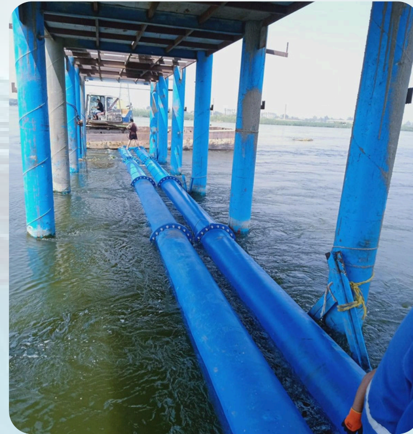
Installation of water station pipes el saf -Installation of clamps and iron beams Pipe installation and connection Installation of valves and filters Installing a weed protection net Underwater concrete crushing Installing pipes on the well and pouring concrete into the water Installation of the external walkway
